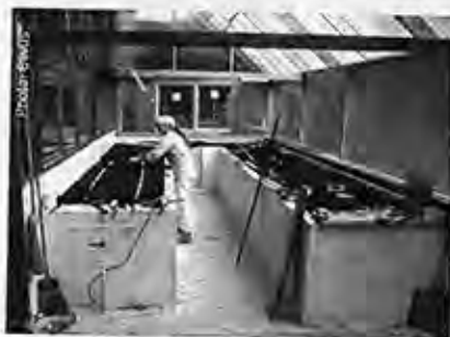
Greenhouse with Clivus infiltration beds in Massachusetts.
