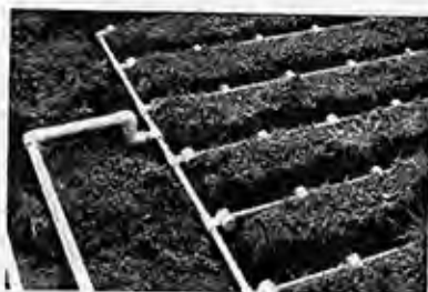
Sand filtered effluent distributed through 1/2" PVC lines with 1/16" holes and emitter shields.
